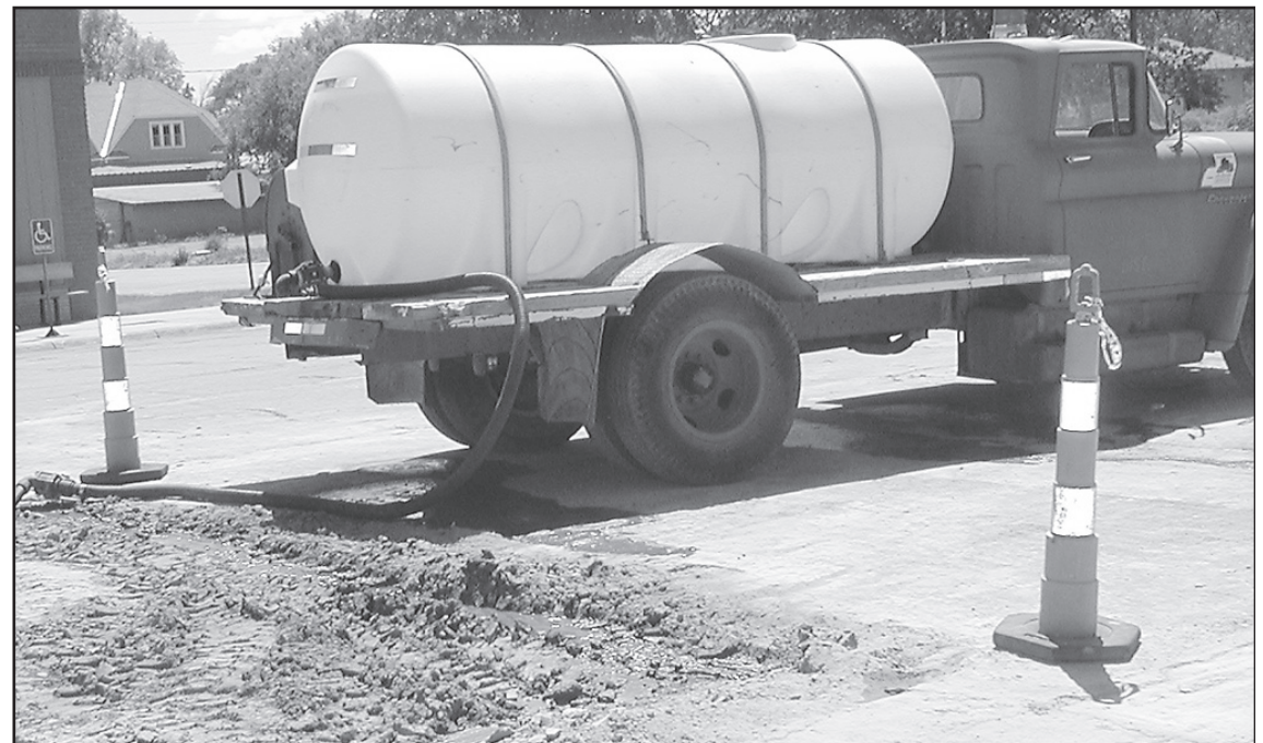
ONCE THE HOLES were filled, the water truck was parked with water slowly running to pack the dirt down before blacktopping the area.
