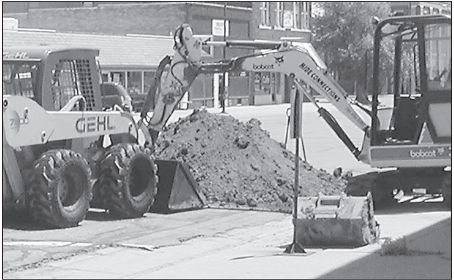
WATER breaks in front of the senior center last week inconvenienced Bird City residents and businesses.
