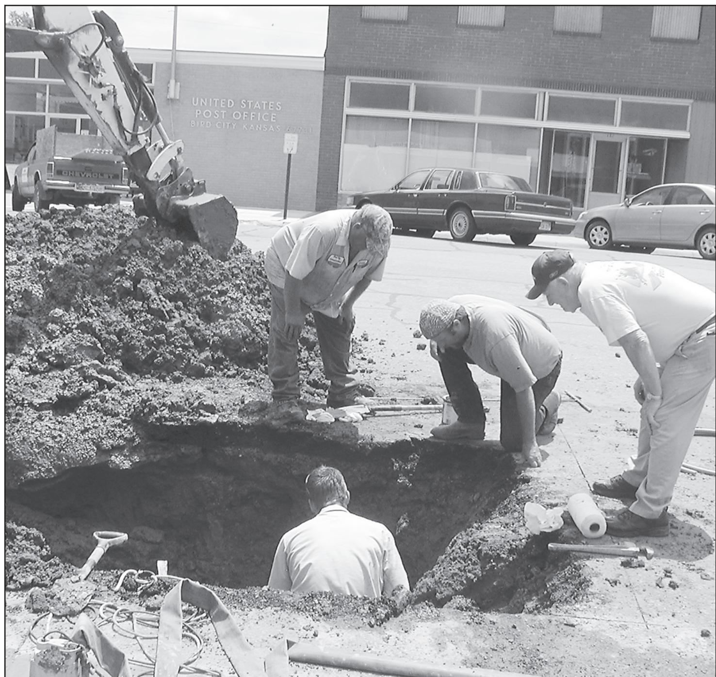
BROKEN PIPES in front of the senior center are being replaced with poly pipe material by Brad Schneider and Russell Jackson, Bird City maintenance crew, and Mike Pochop from Atwood. Terry Burns is checking it out. Times staff photo by Norma Martinez
