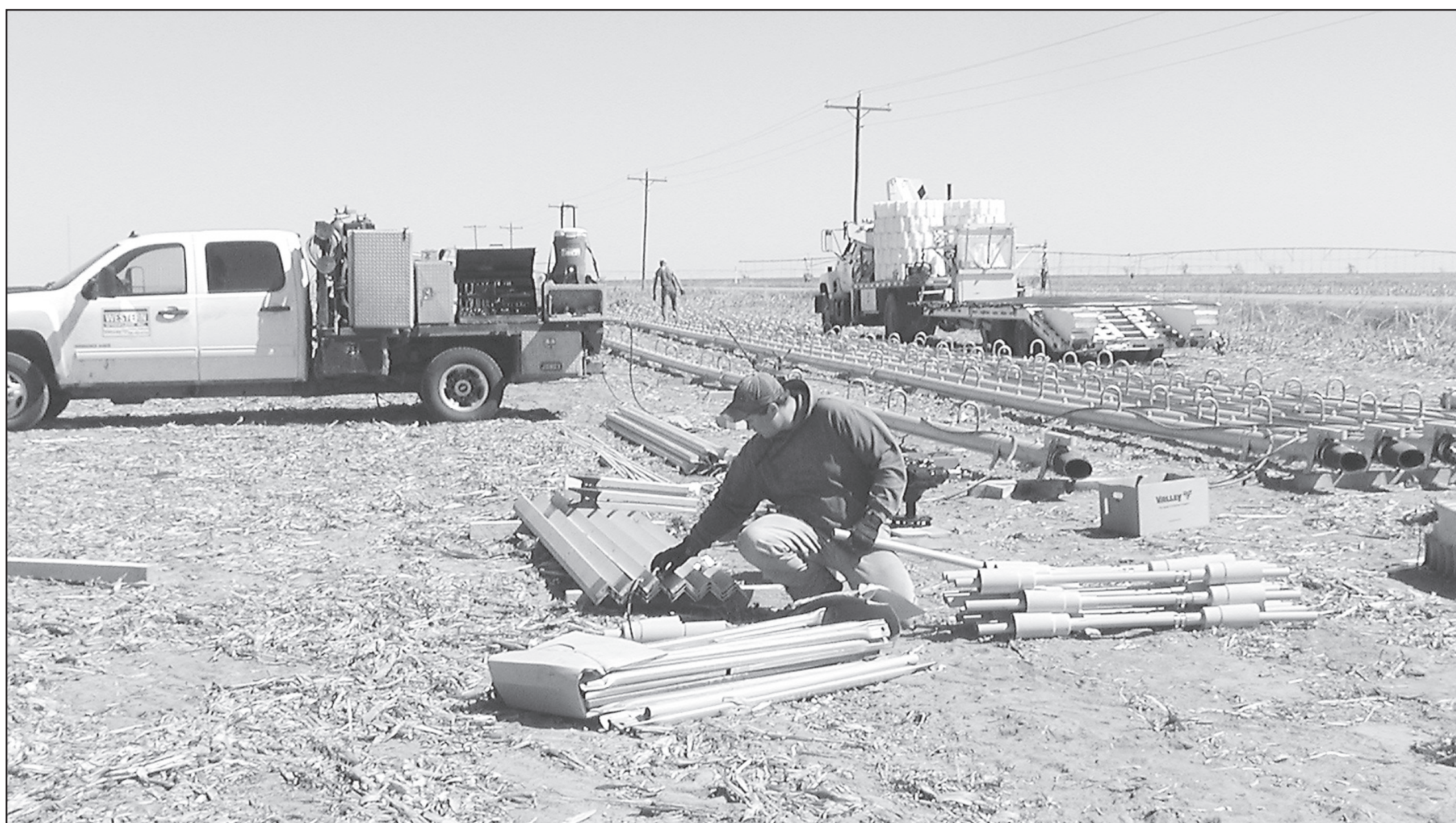
WESTERN SPRINKLERS employees Mike Odoherly and Taylor Finley install a sprinkler system on land owned by Douglas Bell near Bird City.
