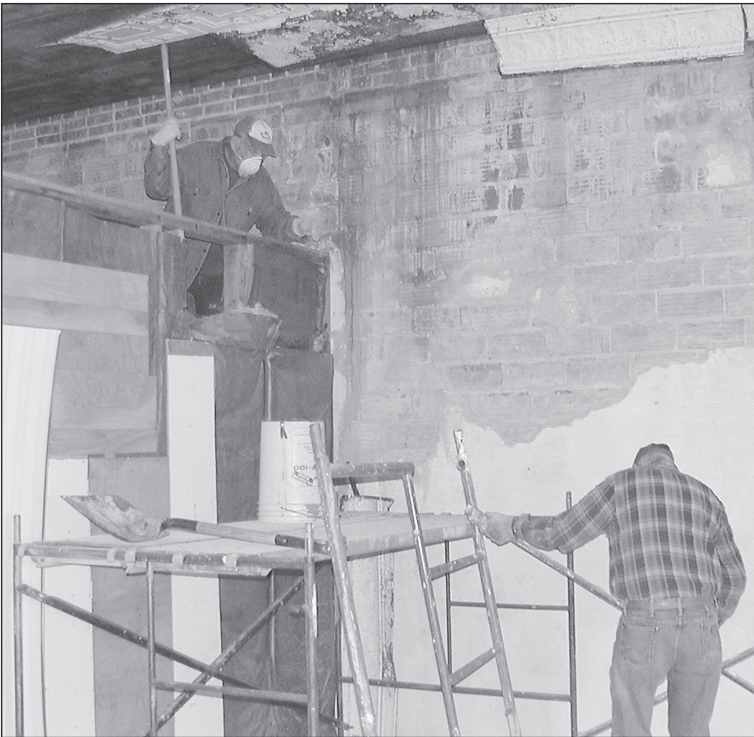
Willy Martinez and Ray Martinez are removing the ceiling tiles and plaster from walls at the Senior Center.
