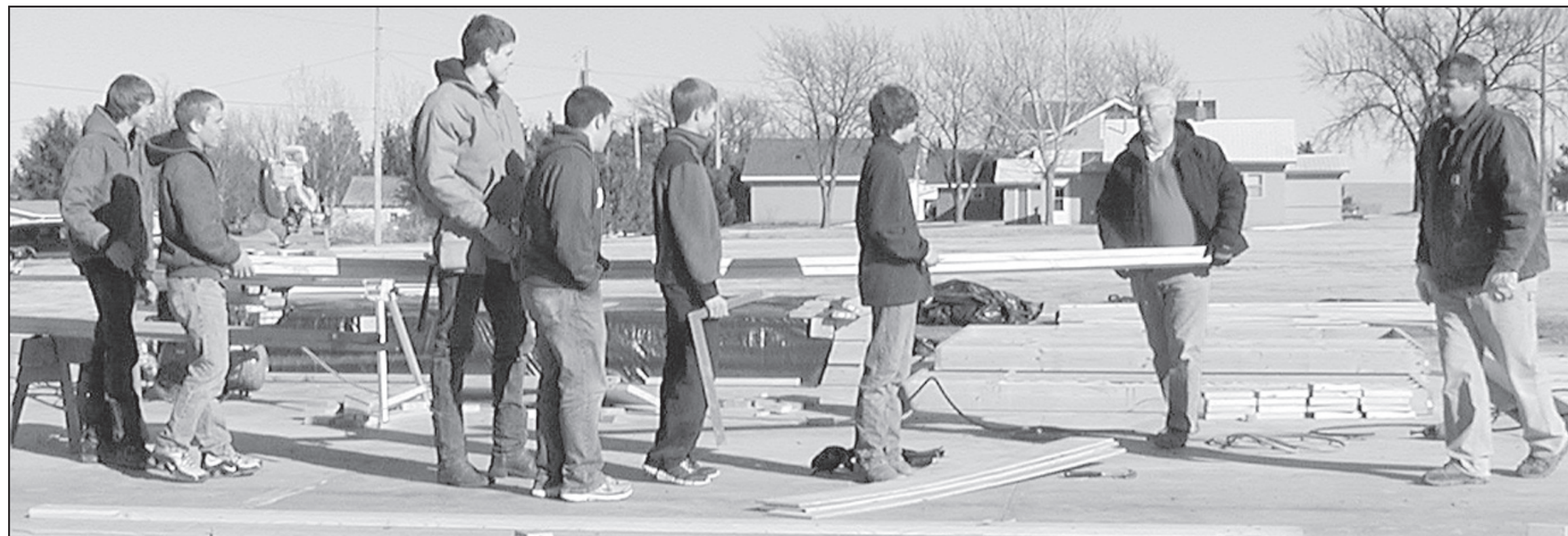
WORK HAS STARTED on the new wellness center. Pictured getting ready to work are student volunteers, Connor Hazuka, Jeremiah White, Josh Keltz, Noah Jones, Ty Carmichael and Casey Vandike. Also helping are Rod Klepper and Dennis Hengen. Times staff photo by Tim Burr
