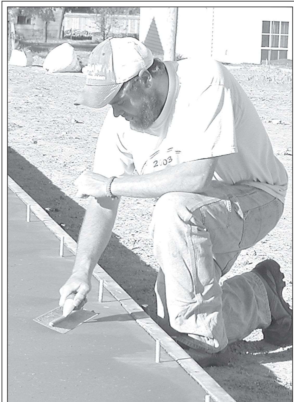
CODY GRAHAM from Shaw Construction Co. is finishing the concrete foundation for the Wellness Center. Times staff photo by Norma
