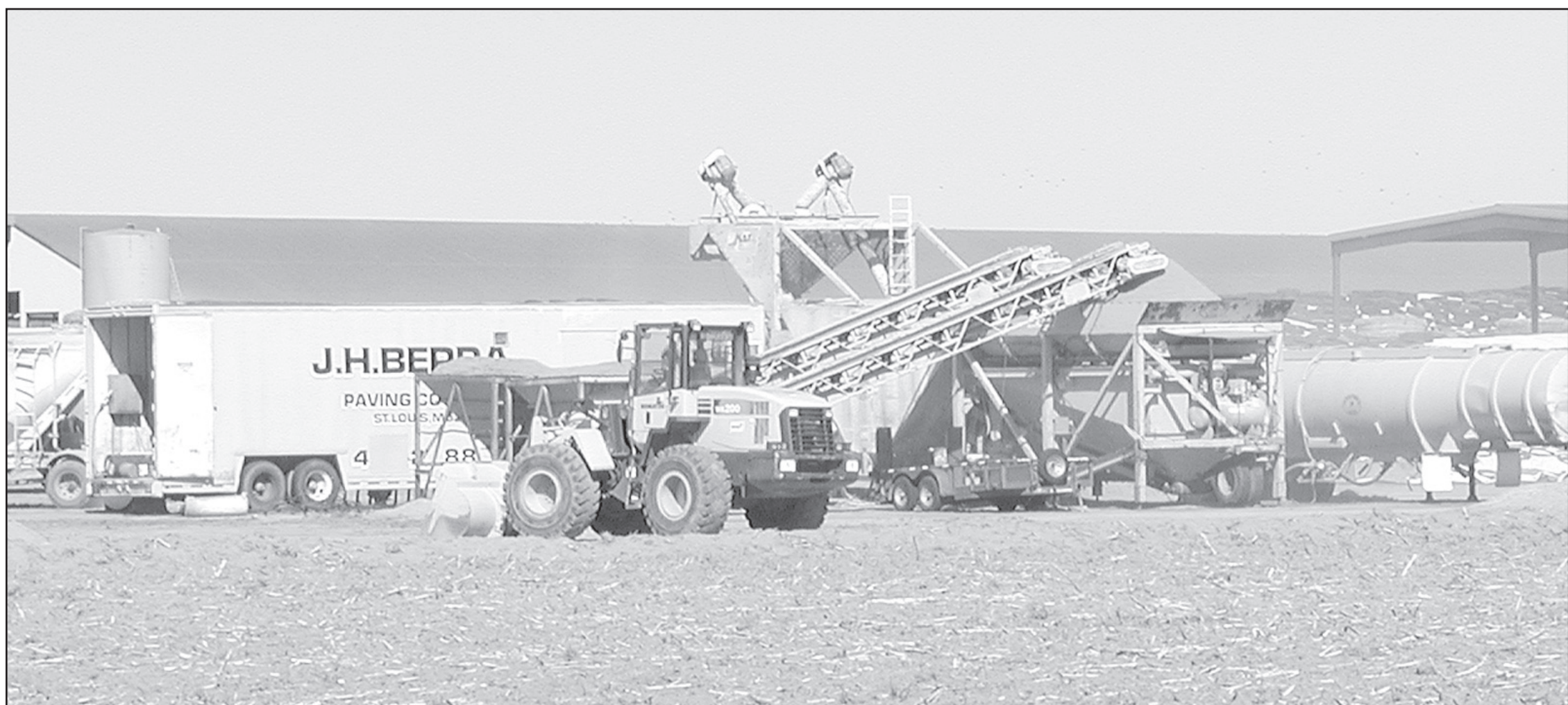
CONSTRUCTION going on at the Bird City Dairy east of Bird City. The cement plant was busy last week as they hurry to get it poured before winter sets in.
