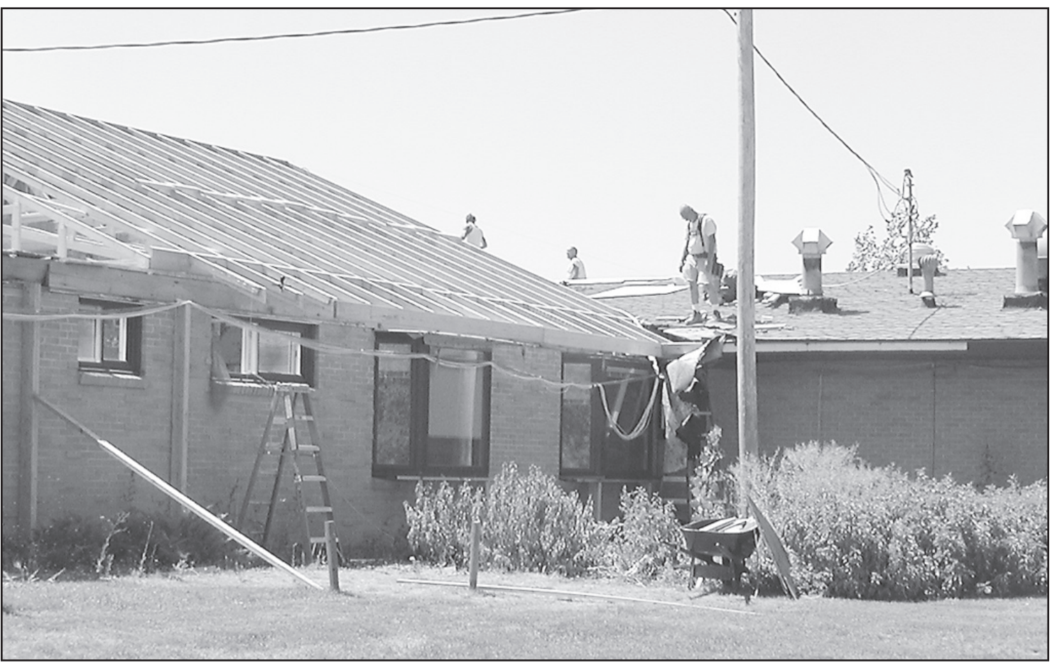
WORK PROGRESSES at the Good Samaritan Village. The underground plumbing has been reconfigured which took some time. Now the roof trusses on the west side are up and the roof is being covered. Getting the new building
