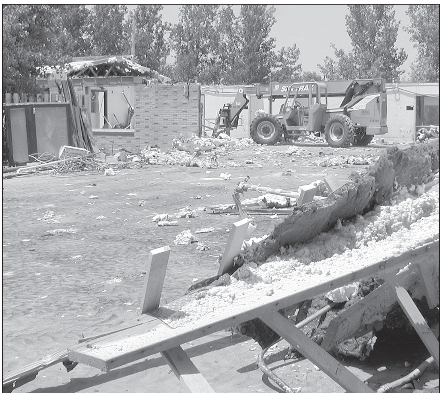
GOOD SAMARITAN VILLAGE demolition is almost halfway done. The completion date is scheduled for December.
