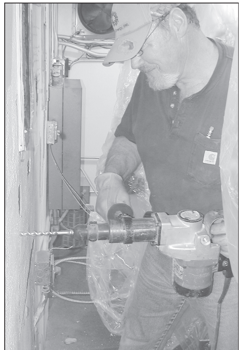
ROGER JENSEN drills a hole in the wall to install the new digital equipment at the theater. The wall is 14" thick.
