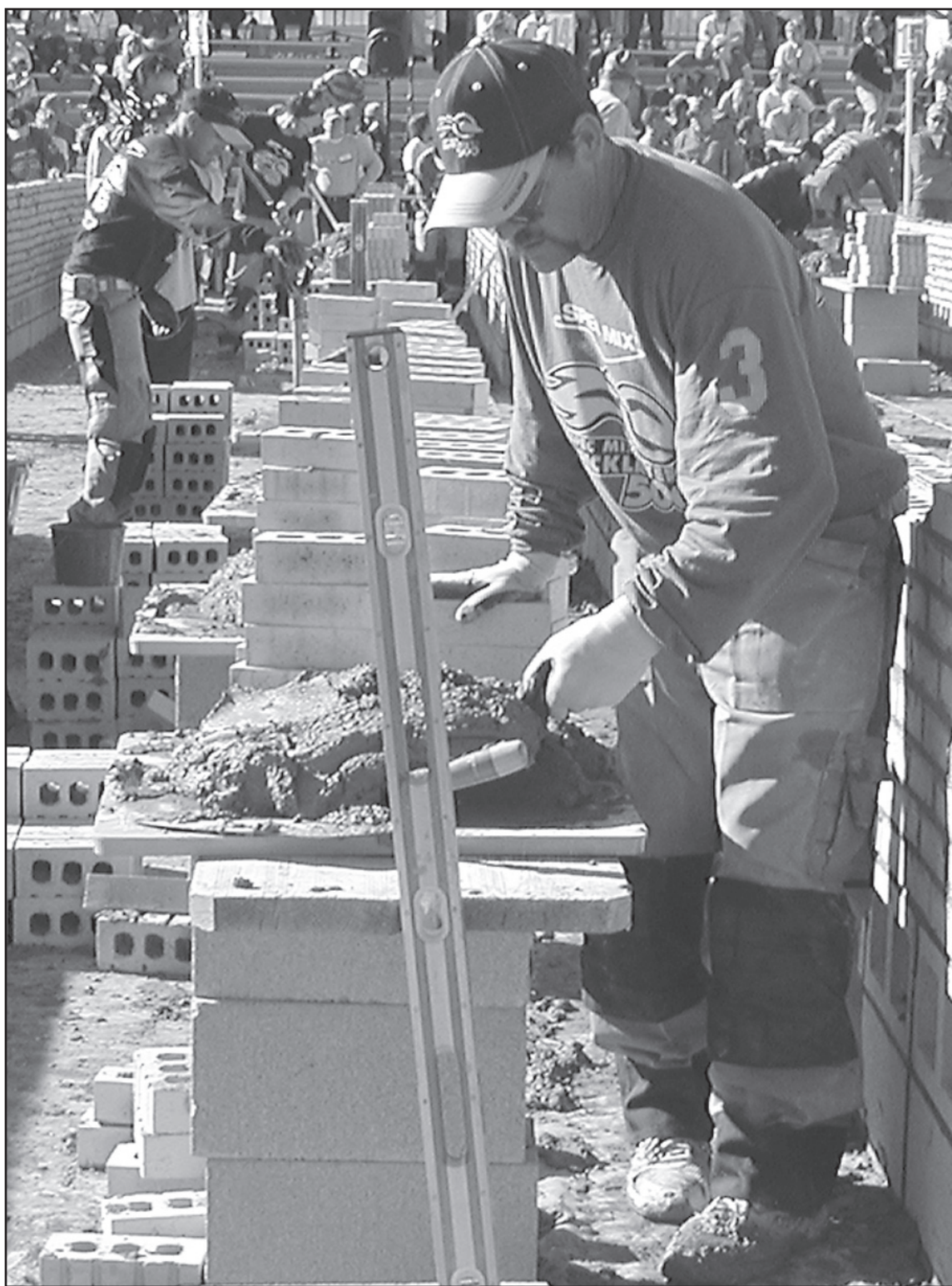
DALE MARTINEZ spreading mud on the last course of 25 foot by 8 inch double wythe wall. Photo by Norma Martinez
