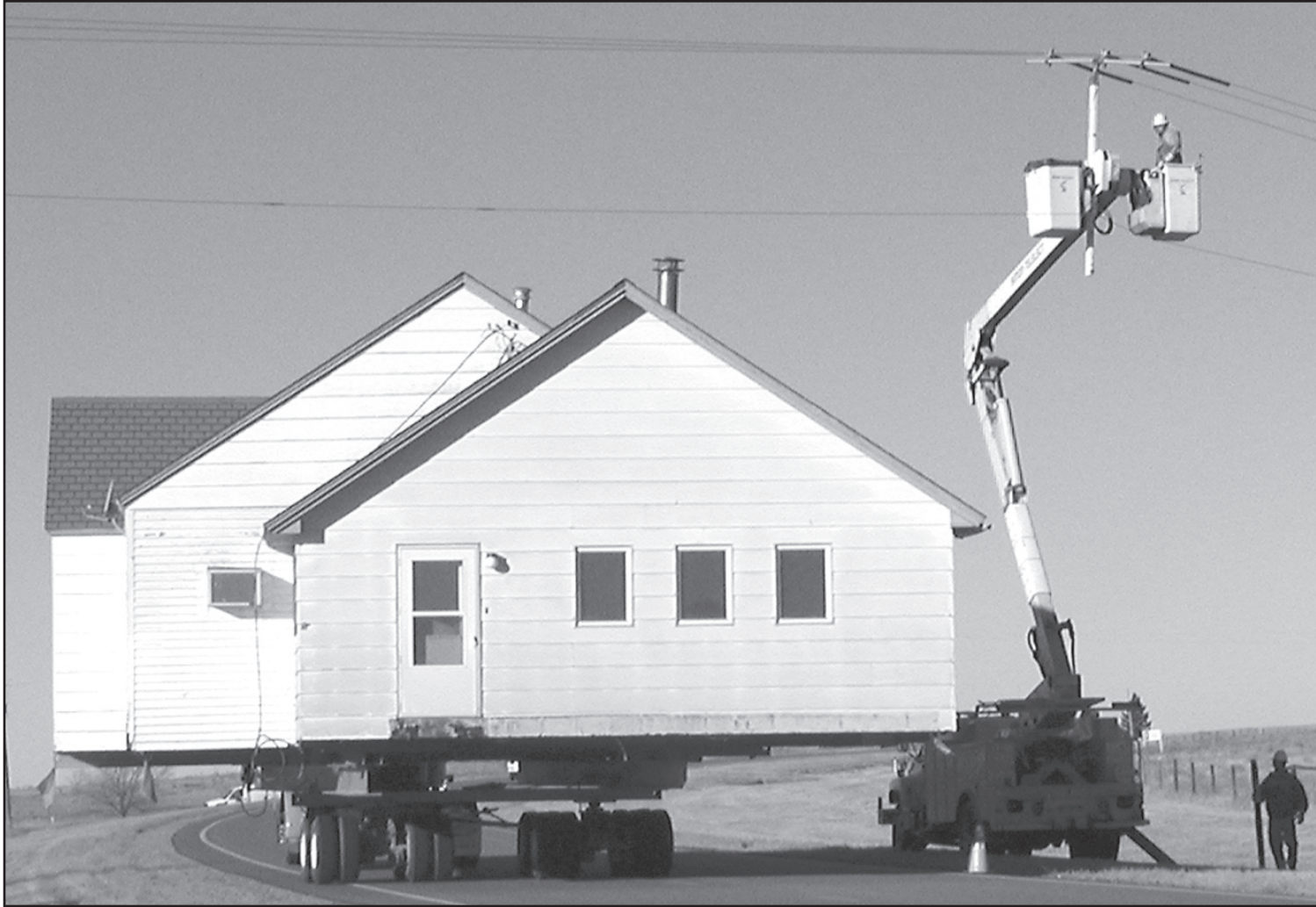
HOLDING UP THE POWER LINES — The crew raises the power lines as they move the house to the Troy and Kary Meyer property near St. Francis.
