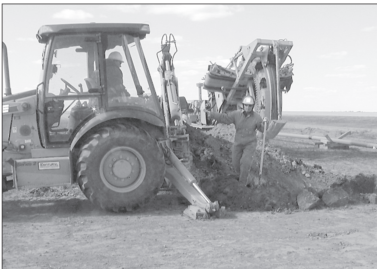
LAYING A PIPELINE , Lester Baker and Joyce McArthur from Wray, Colo., work on a 21 mile gas line. The work is being done along Highway 36 from east of St. Francis to six mile north of Bird City. Times staff photo by Norma Martinez.
