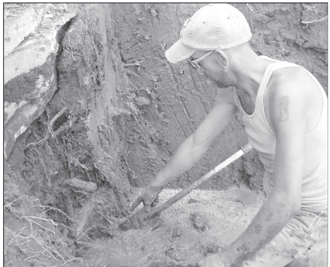
ERIC BARTELS, city worker, points to the water leak found while demolishing a house on Cave Avenue.
