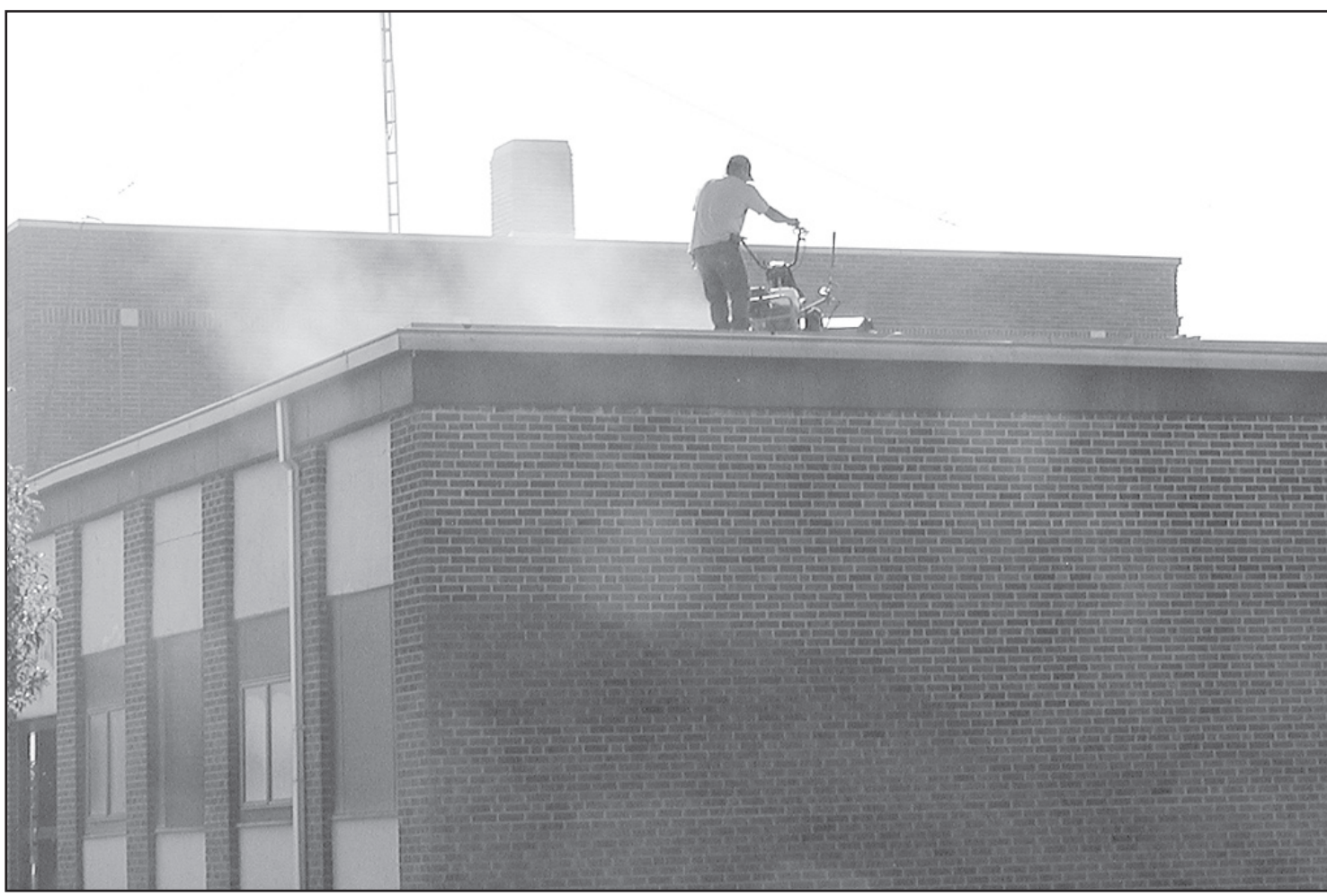
THE LAST WEEK of July when the temperatures were in the high 90s, workers were on the roof of the elementary school building. Striping it in preparation for a new roof. The first day of school is Aug. 17.
