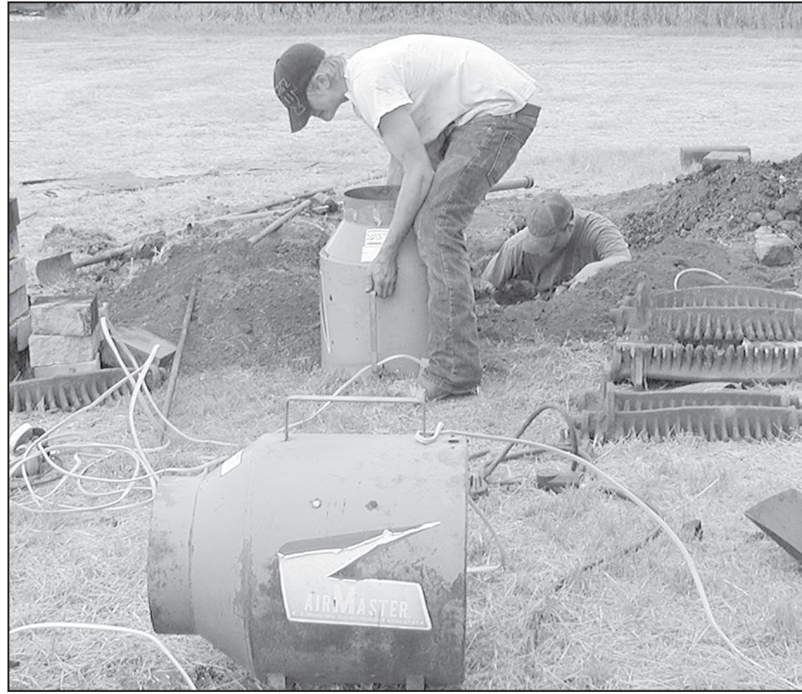
TRYING TO MAKE repairs, David Michaelis (left) and David Burns work on fire pit. It was hoped that the heat would help to straighten some metal pieces.
