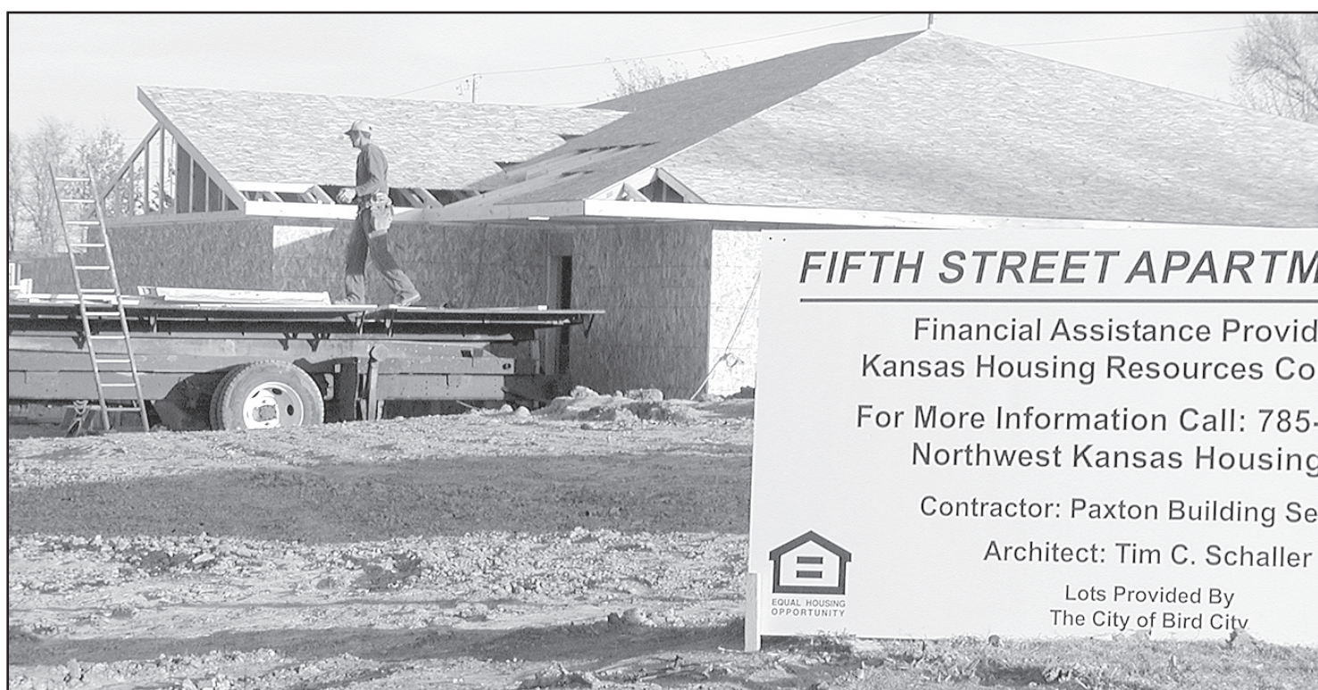
FIFTH STREET APARTMENTS are coming along and will soon be ready for occupants.
