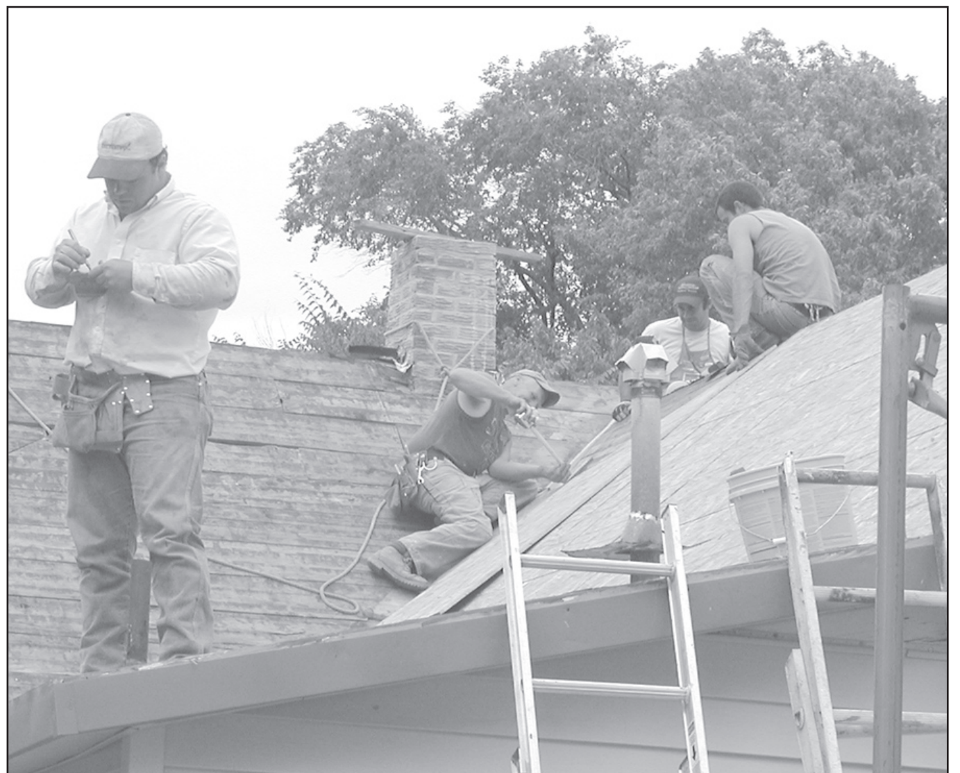
BIRD CITY RESIDENTS SHOWED UP for a couple of work days at George Bandomir's home to repair and replace his roof. It was a team effort with workers on the roof hammering, workers on the ground sawing and preparing supplies, and workers stopping by with lunch to keep it going smoothly.
