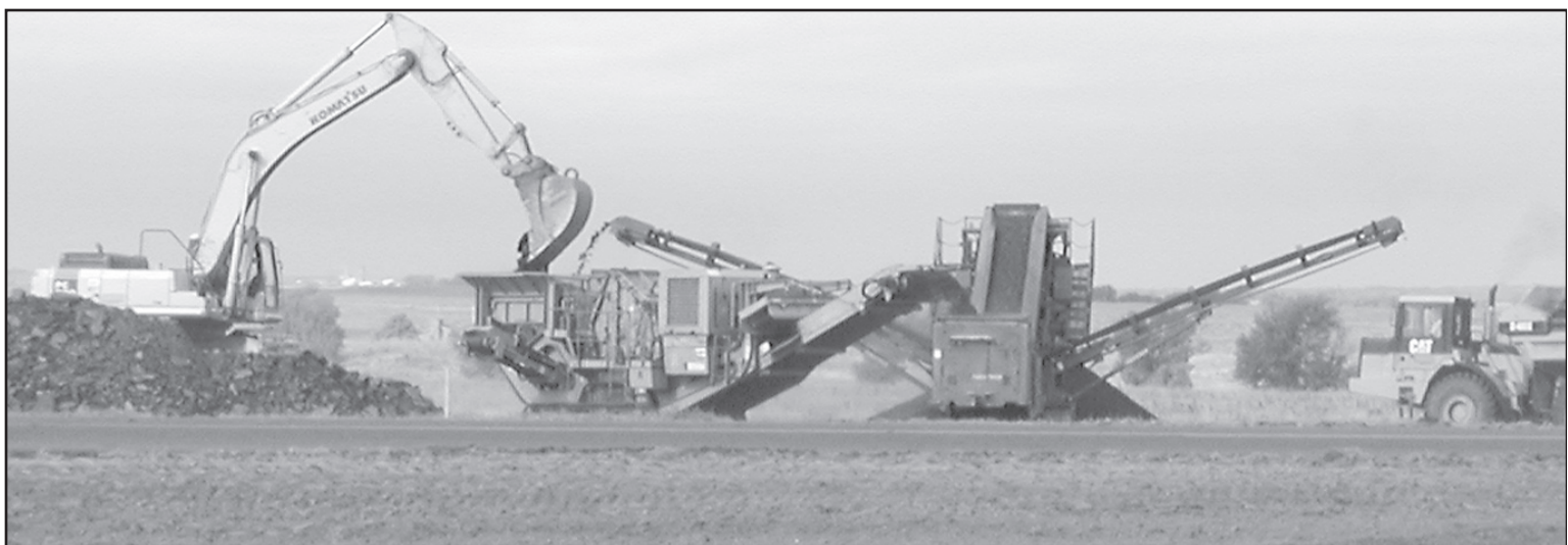
WORK ON THE AIRPORT RUNWAY at the Cheyenne County Airport in St Francis began on Monday and will continue until some time in October. Herald staff photo by Karen Krien
