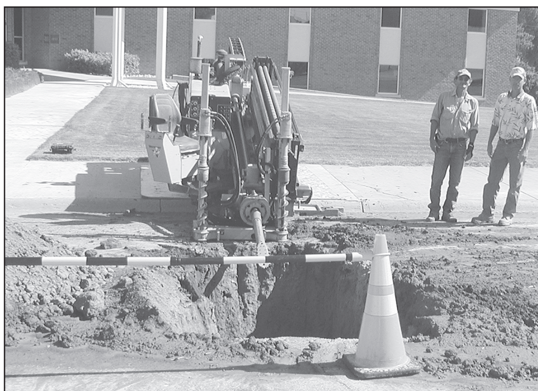
WHERE IS THE WATER GOING? H&H Sprinkler company is in town digging holes and looking for water leaks.
