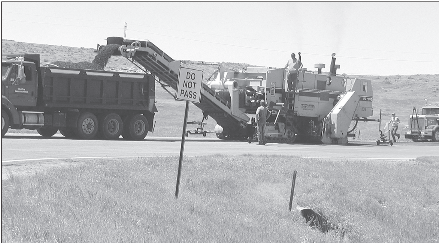
HEAVY EQUIPMENT works to repair K-27 north of St. Francis. The crew is making a real effort to be done before harvest.
