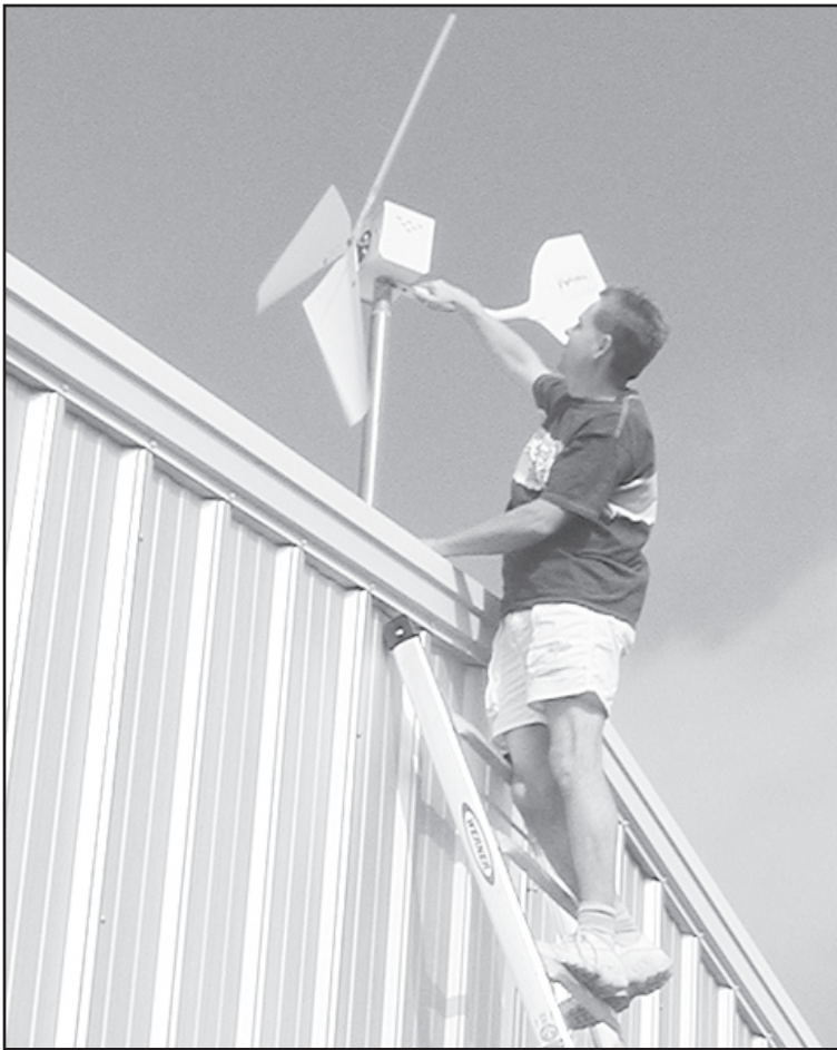
HARNESSING THE WIND! Marlin Queen positions a wind turbine on top of a building. Times staff photo by Karen Krien
