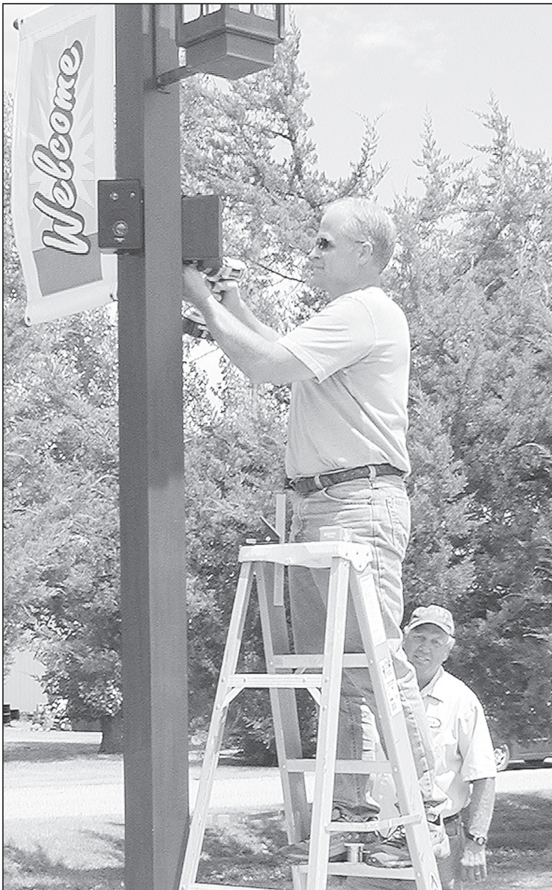
WADE CARMICHAEL INSTALLS new speakers at the Van Doren Park. Assisting him is Brad Schneider, city maintenance.
