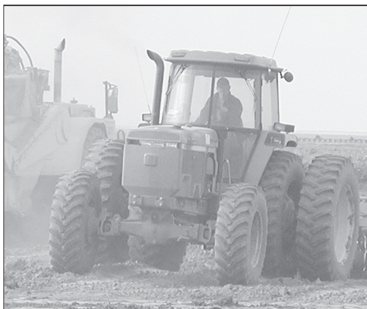
MOVING THE DIRT right along side of the big tractors, this John Deere gets the job done digging the lagoon.
