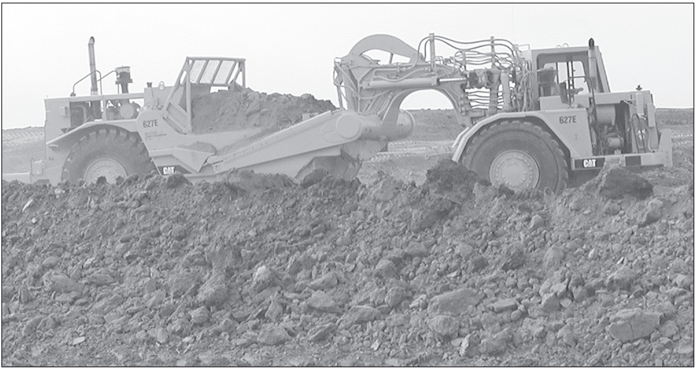
RAIN SHOWERS DID not slow down the construction of the lagoon in Bird City. Several earth movers working together to pile up the dirt around the lagoon to create a berm. It is only the first step in getting this project completed.
