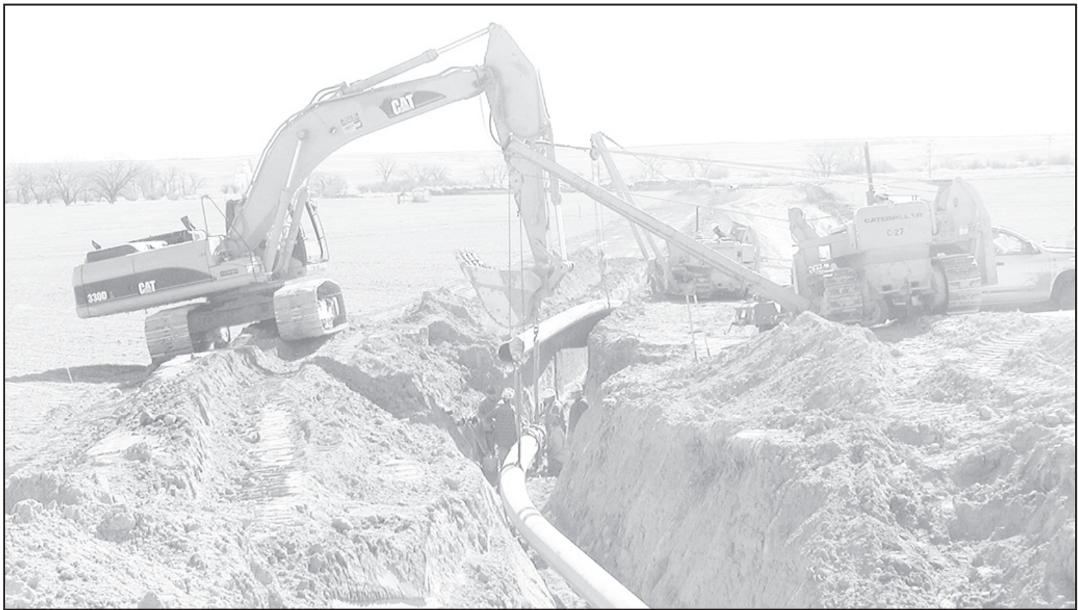
LOWERING A 20-FOOT SECTION of steel pipe to carry natural gas — the pipe is being laid across Cheyenne County. This line is being put in out north of U.S. 36. Times staff photo by Casey McCormick
