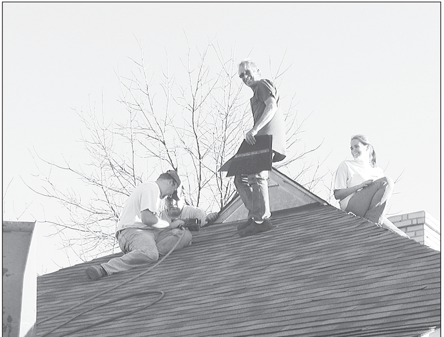
REPLACING OR REPAIRING worn out roofs is a cost effective plan to reduce future heating and cooling bills. It also helps when family members pitch in.
