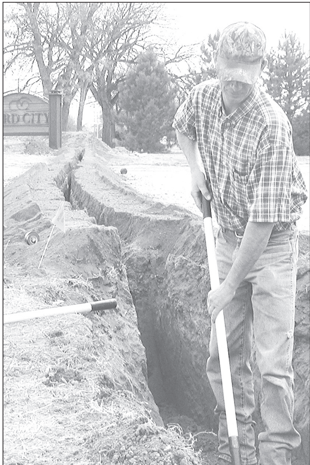
WORKER, Troy Horinek from HHSprinklers, Goodland, digs the trench for the electric cables that will soon be lighting up the Bird City welcome sign. Times staff photo by Linda Schneider
