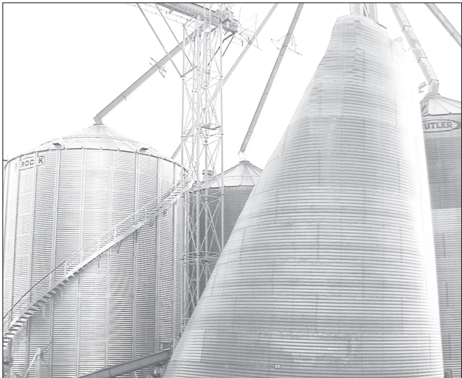
ONE OF the grain bins at McDonald Equity was damage by the Microburst that went through.
