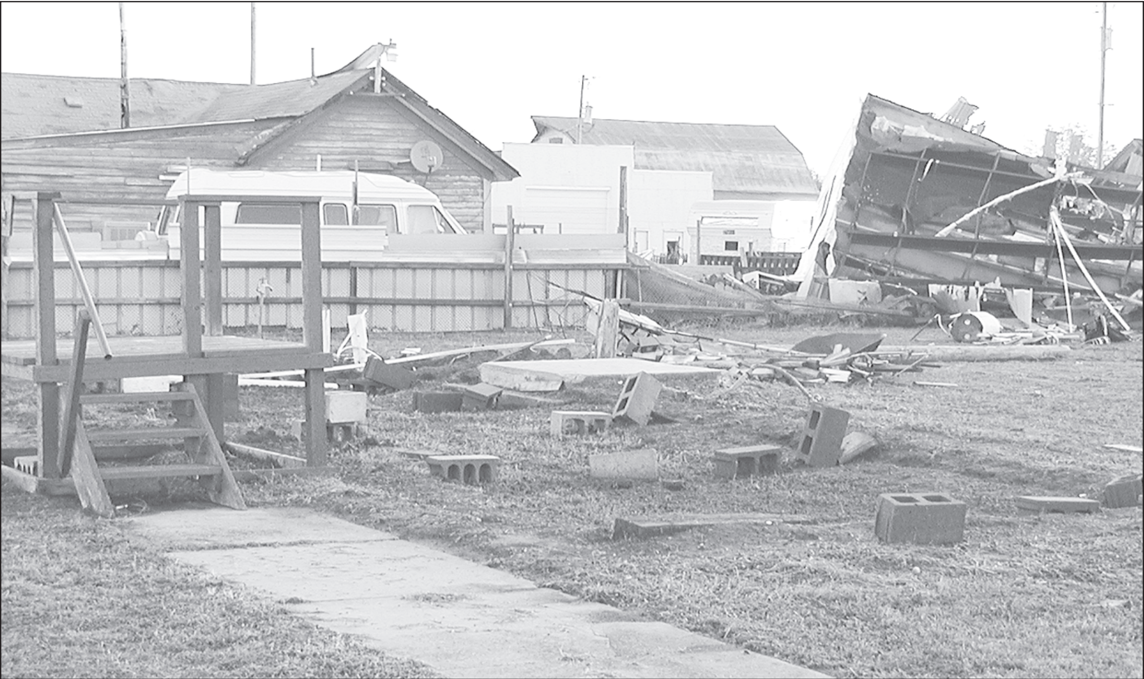
THE TRAILER HOUSE belonging to Joice Pedersen is gone with only the steps still intact. No one was in the home at the time of the storm on Thursday night.
