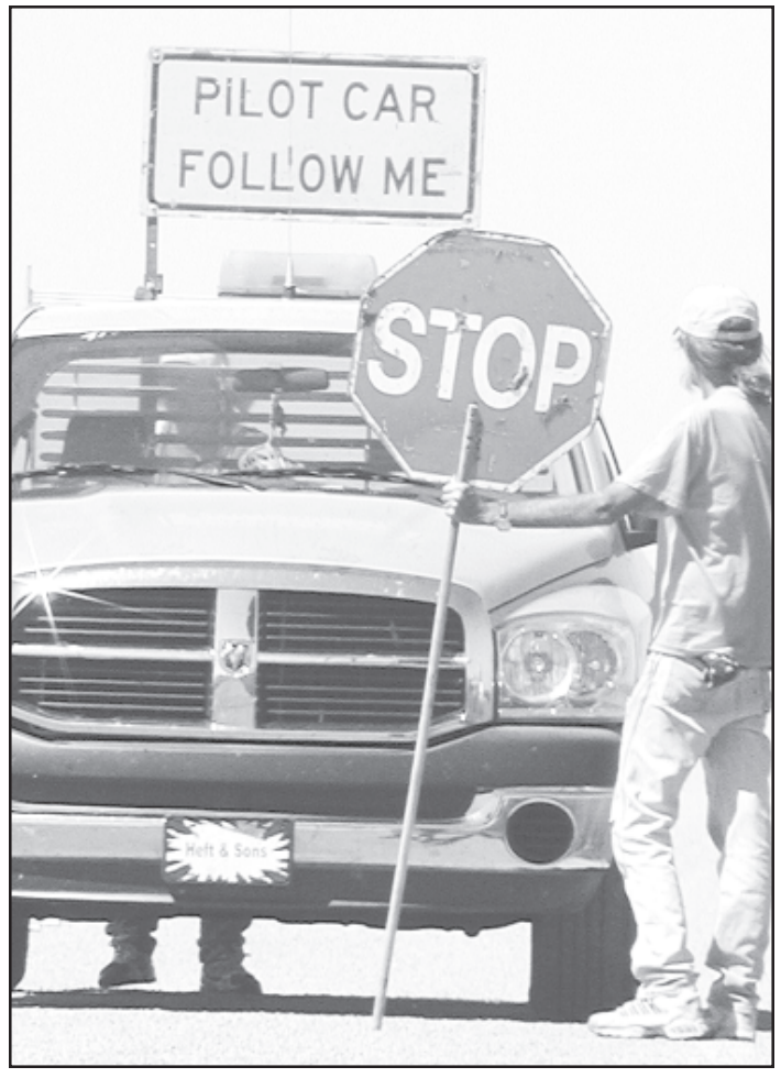
ONE WAY TRAFFIC will be found on K-161 as the highway is resurfaced. Chris Zulick was stopping traffic and said the work should be done by the end of the week. Herald staff photo by Karen Krien
