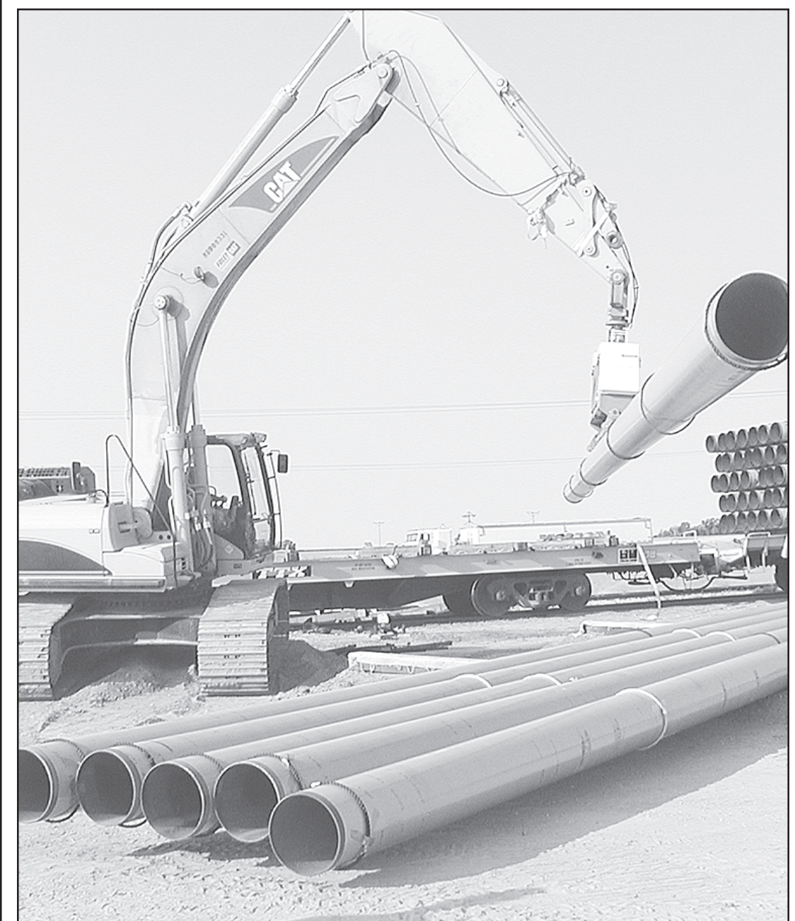
16 INCH PIPES for a natural gas line are unloaded from rail platforms in Bird City. About 40 platform cars of pipe were also delivered to McDonald. Times staff photo by Casey McCormick
