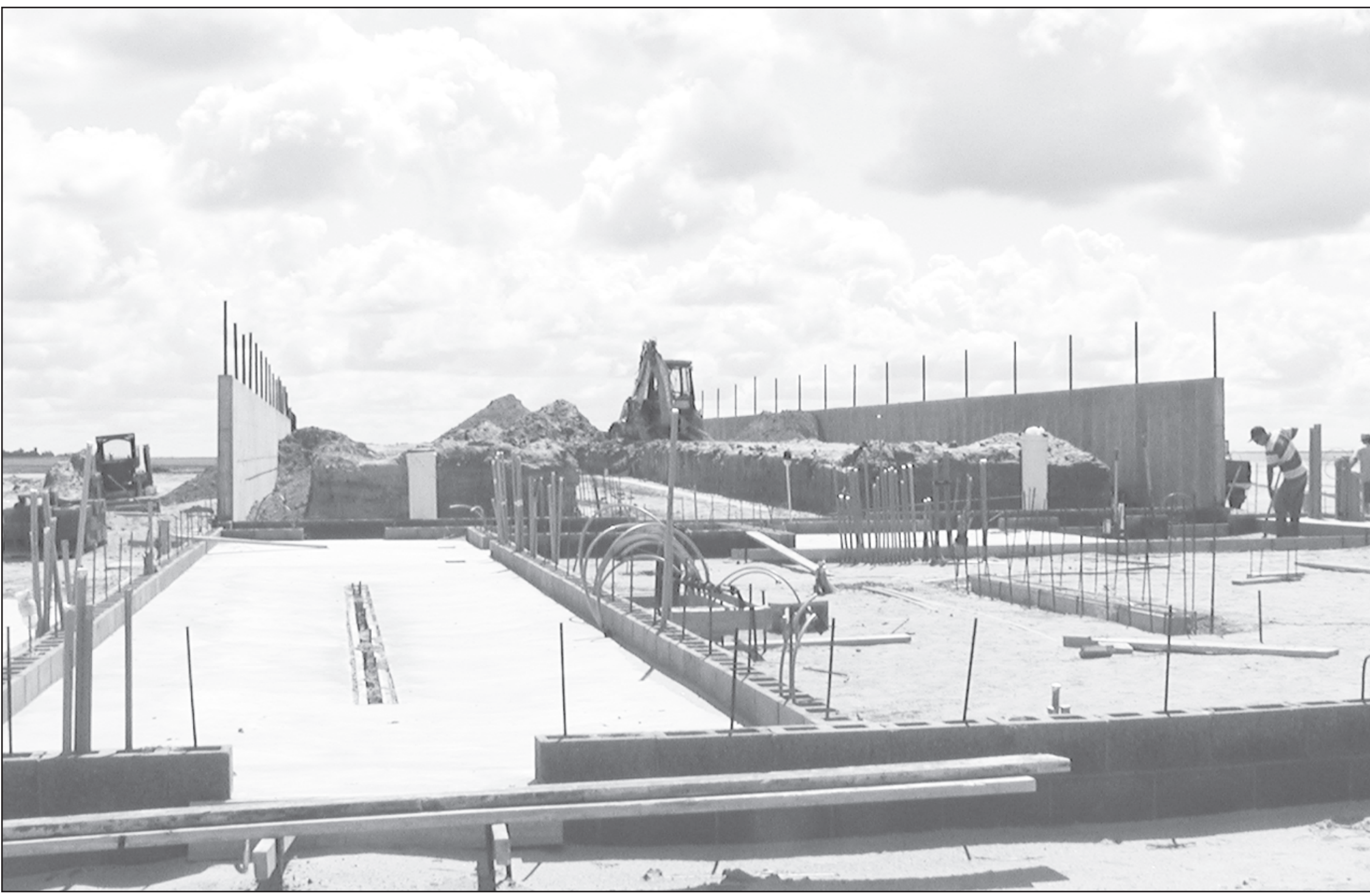
Progress on the dairy is moving right along. Gary Wilhite, construction manager reported that by next week this milking parlor should have a metal structure covering it. The dairy plans to begin milking around September first. Times Staff Photo by Melinda Basnett
