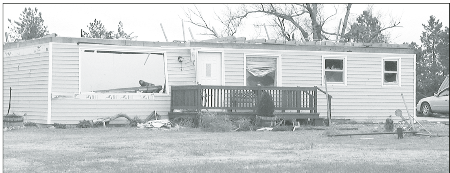
John and Maria Kamla home with the roof ripped off. Photo by Melinda Basnett
