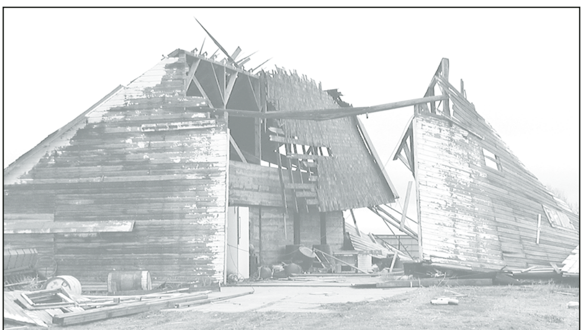
Most of the Oscar Johnson barn was gone.
