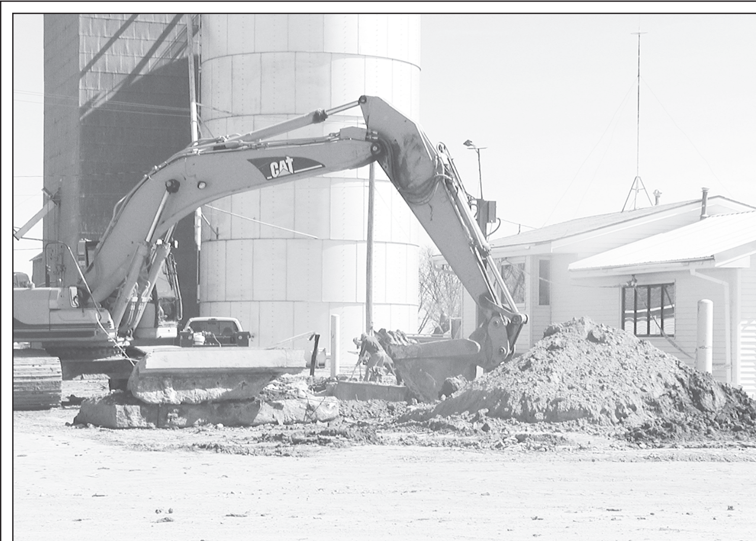
DIGGING OUT the old scale at McDonald Equity, crews are working to enlarge the scale to accomodate the larger trucks that farmers use today.
