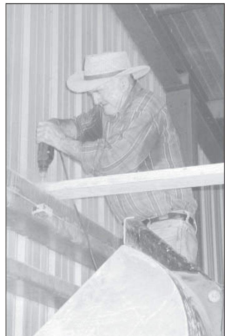
GETTING READY —Larry Henry is busy making repairs and improvements for the 2004 Thresher Show. Times staff photo by Casey McCormick
