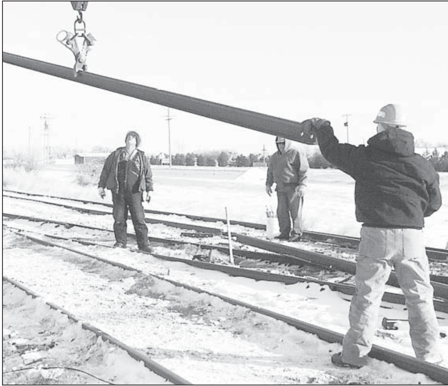
WORKERS FOR THE Nebraska-Kansas-Colorado Rail Road fight the elements to repair a section of track damaged earlier by a derailed tank car. Freezing temperatures and bitter winds made the men from Nebraska earn their wages.
