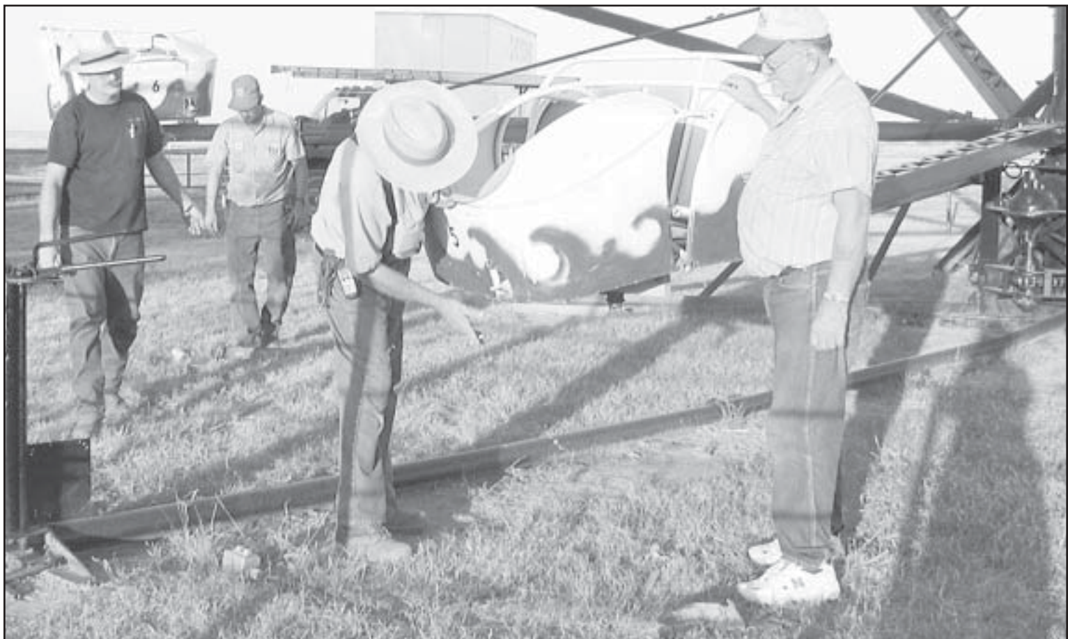
NEW OCTOPUS RIDE will be ready for action at the Cheyenne County Fair Aug. 6-9. Pictured (l to r) are Amusement Authority member Greg Walz, Bill Ehrman, Sam Miller and Marvin Confer. The ride needed repairs, painting and greasing before it was ready to go.
