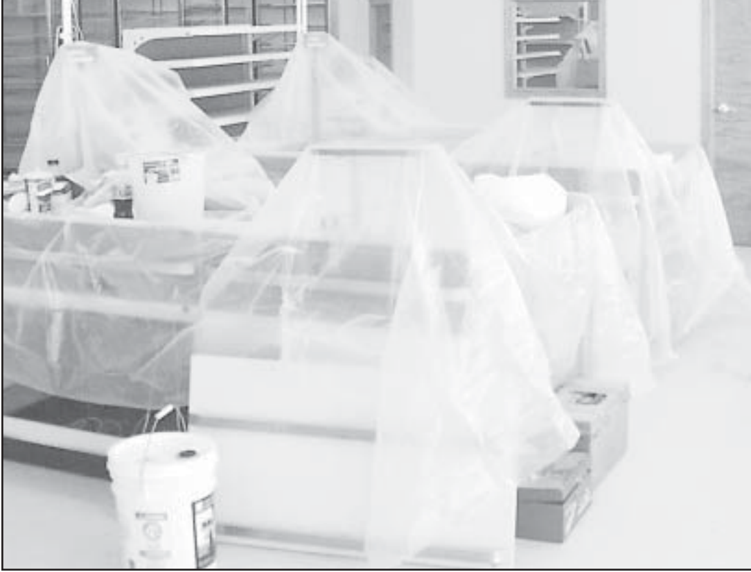
DUST COVERS PROTECT electronic scanners and registers soon to operate in the renovated Bird City grocery store. Times Staff photo by Casey McCormick
