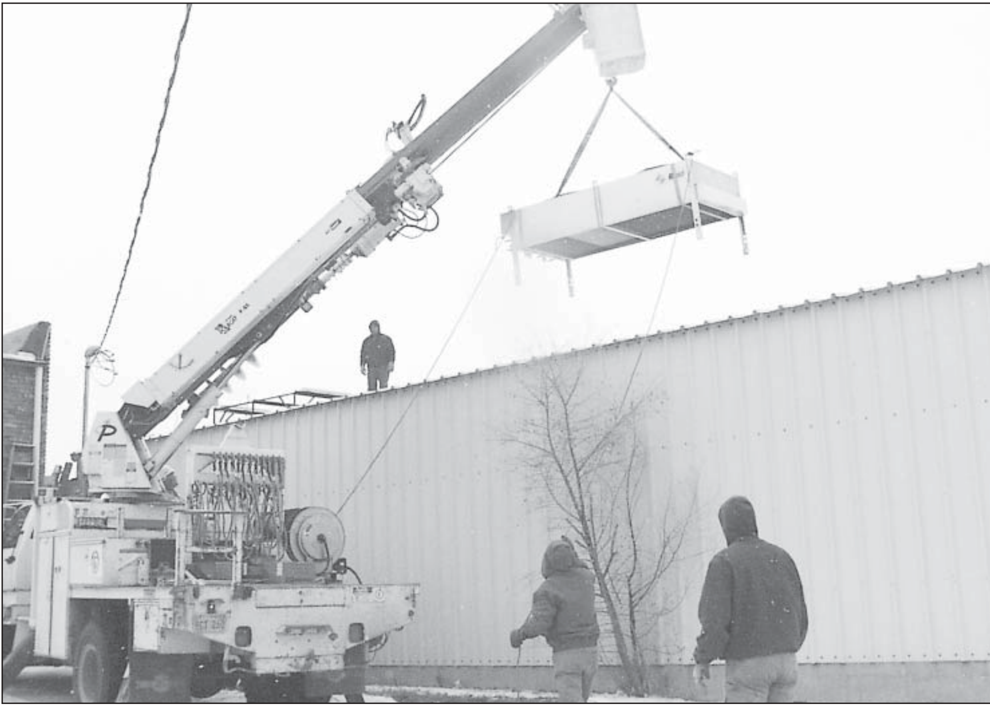
A CONDENSER was placed on the roof of the grocery store as the remodeling is progressing at a steady pace.
